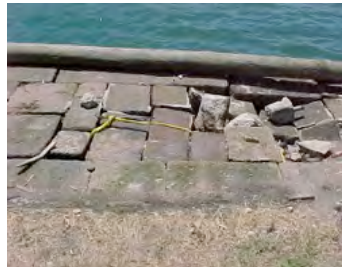
Collapsed section of old wall near Officers Quarters.
