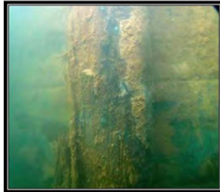
Copper sheeting on tarred wood piles over 200 years old.
