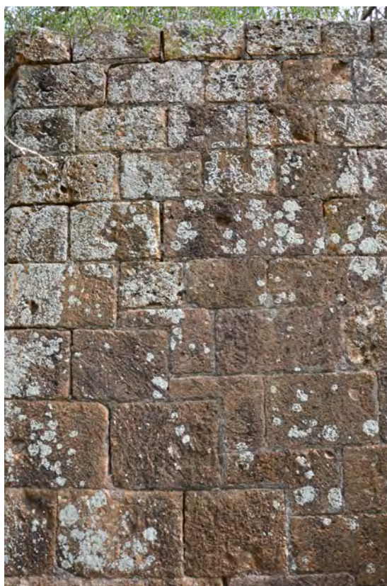
Figure 62. North Bastion Wall at Dow's Hill Fort in an excellent state of repair
